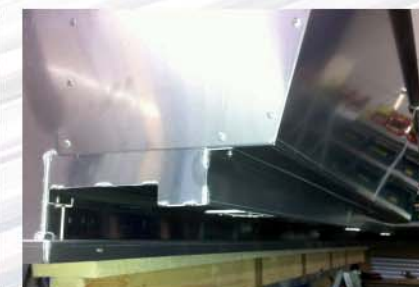
The side boxes have got a rain gutter
