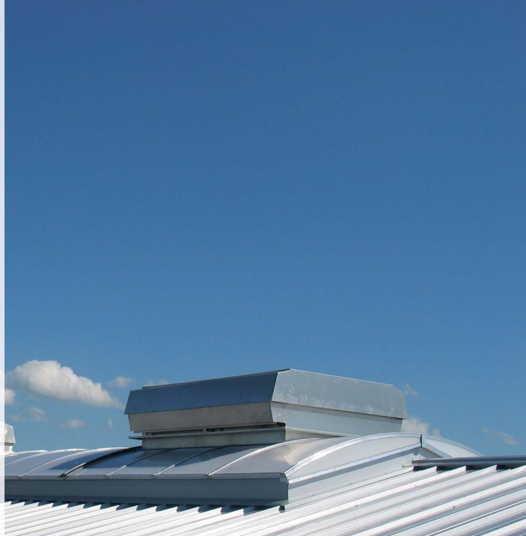
The SHE and ventilation systems may also be integrated into a continuous skylight system, which allows daylight to enter the building and thus decreases operating
