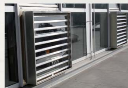
SMOKEJET in vertical glazing
