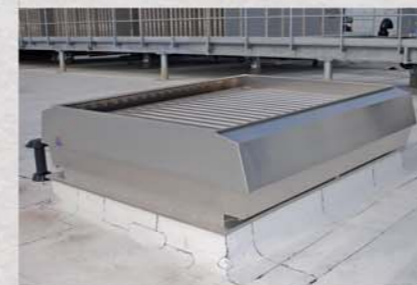
Stand-alone unit on a factory roof
