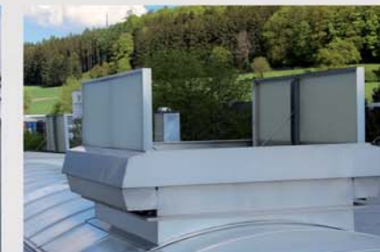
MEGAPHOENIX on a skylight
